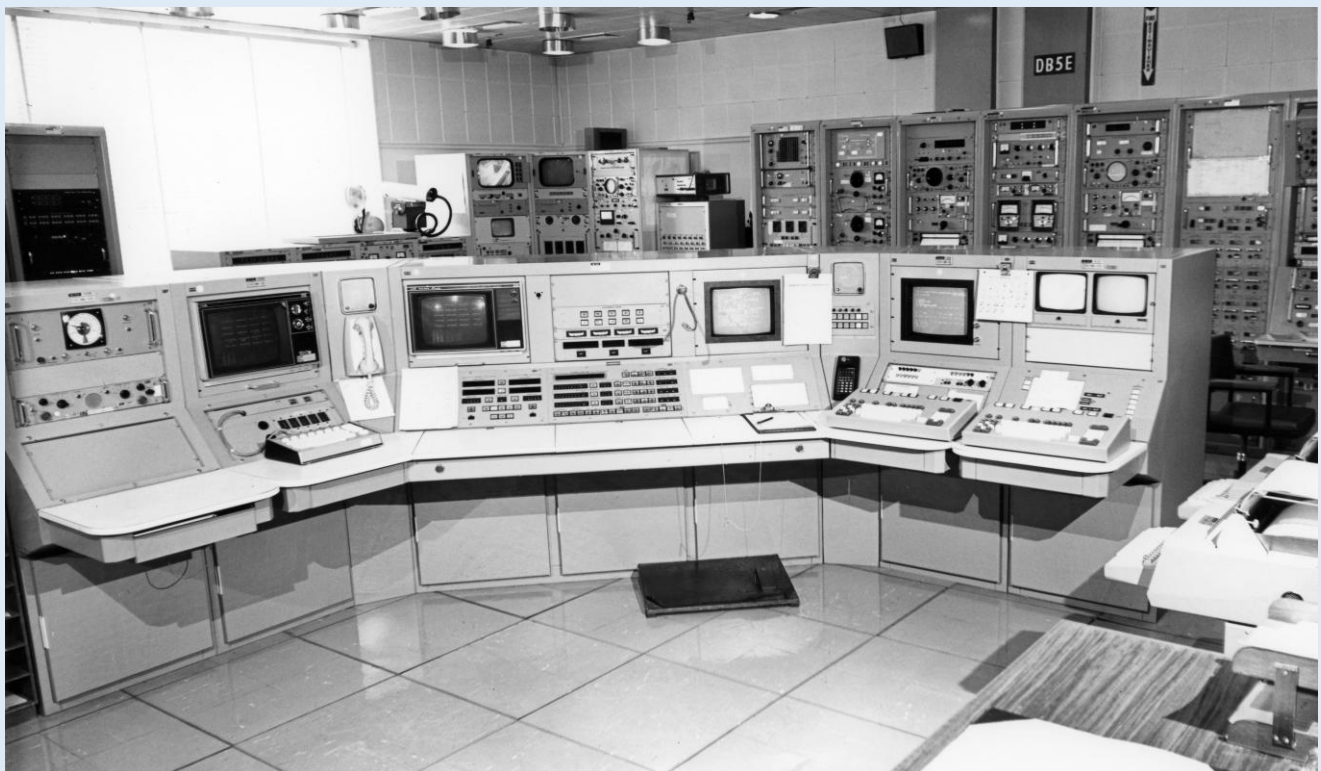
Below: The expanded Operations console in its new location.
